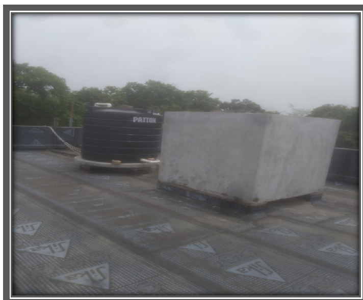
Fig. 10 : Drinking water storage tank
